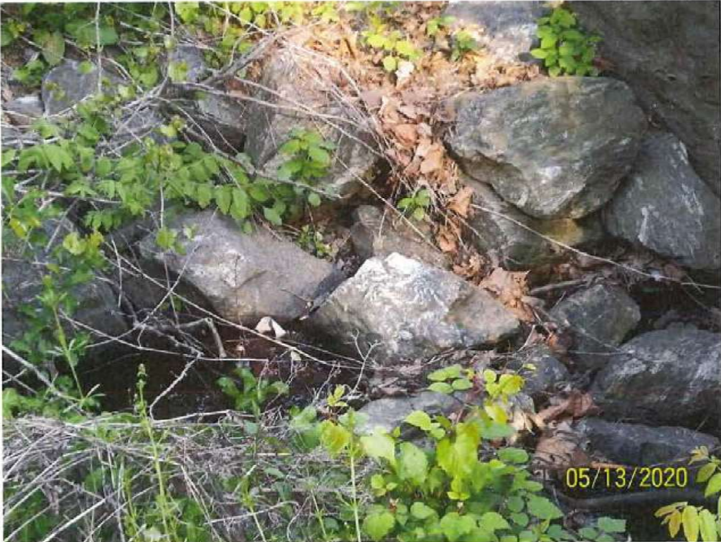
Figure 4. Flowing water observed.
