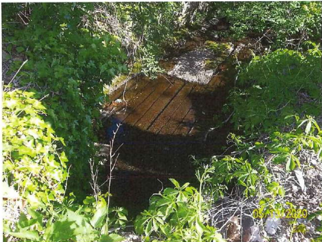
Figure 24. Water flowing out of culvert.
