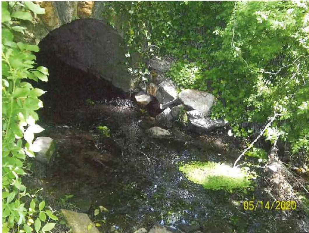
Figure 9. Culvert on the south side of E Rose Valley Road. Tributary continues.
