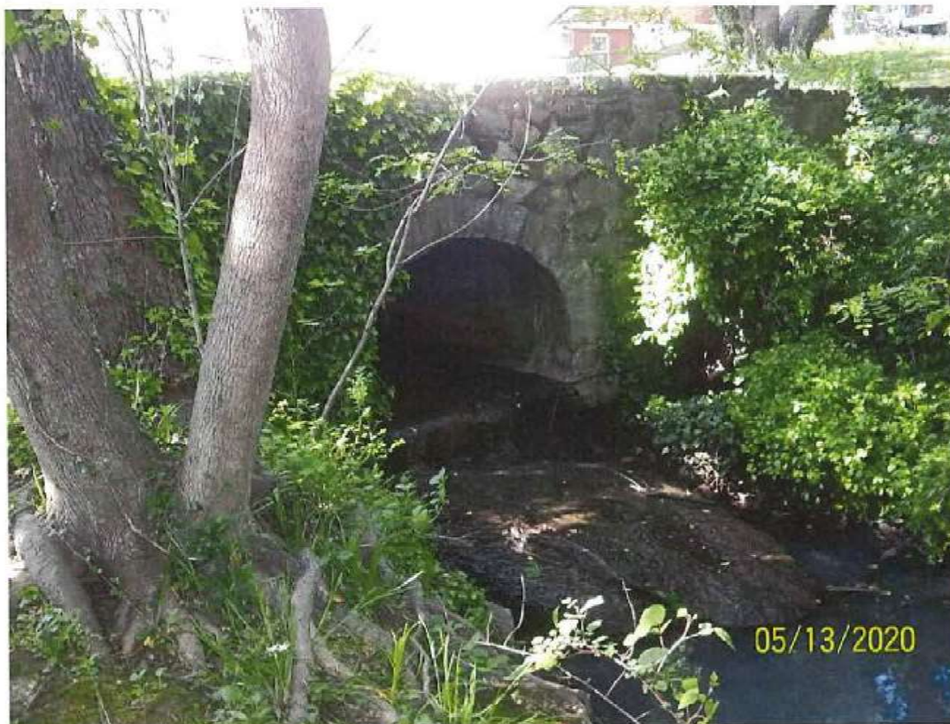
Figure 3. Culvert under driveway from Figure 2. Flow first observed here. Beginning of Tributary.
