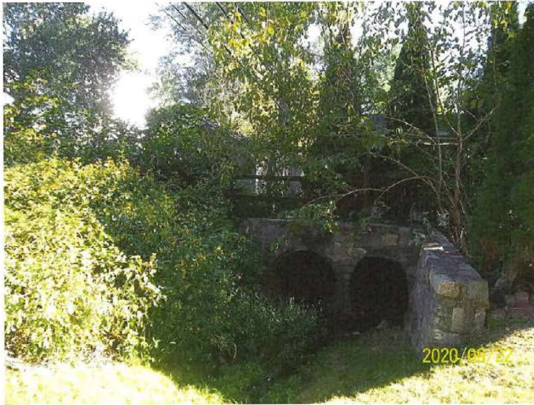
Figure 7. Headwall in the backyard of 428 Palmers Lane where tributary goes underground to cross East Rose Valley Road.
