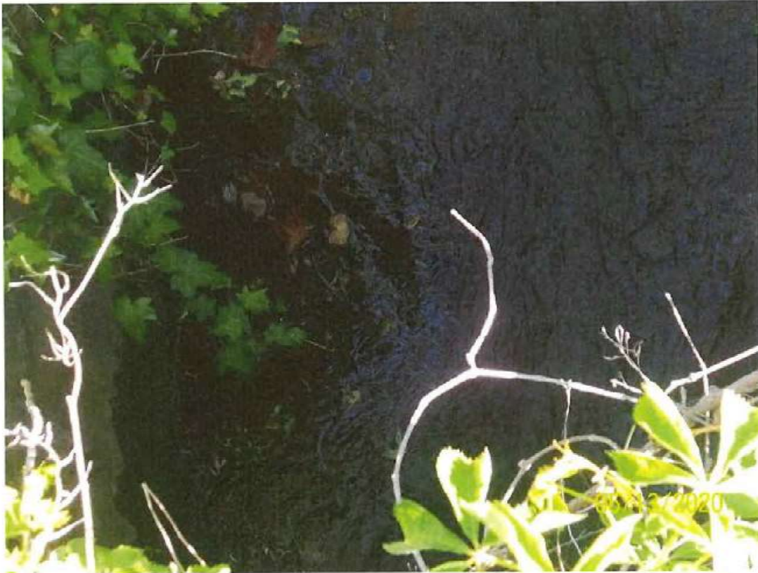
Figure 23. Water flowing out of culvert.
