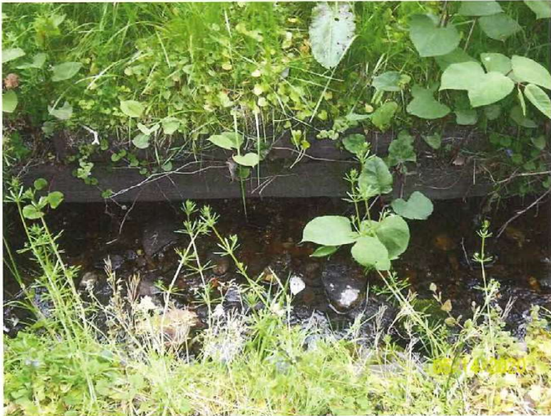
Figure 15. Flowing water observed.
