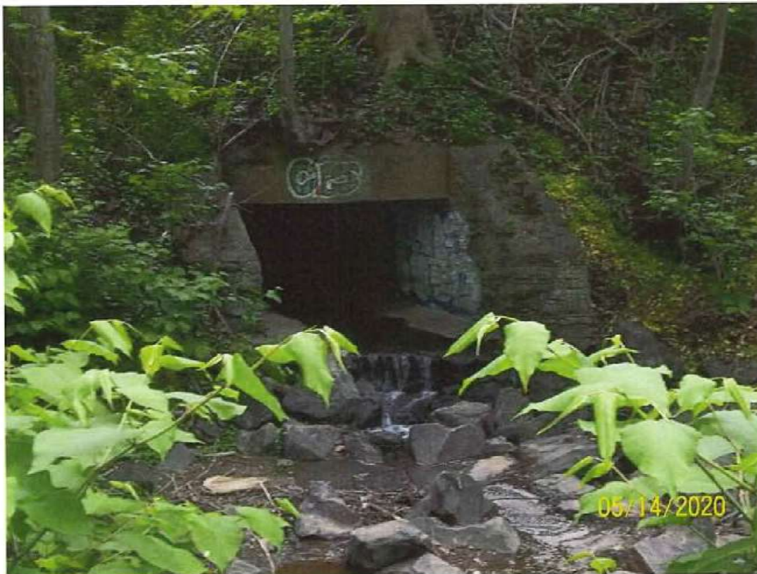
Figure 29. Pine Ridge Run resurfacing from culvert on the other side of the trolley tracks.
