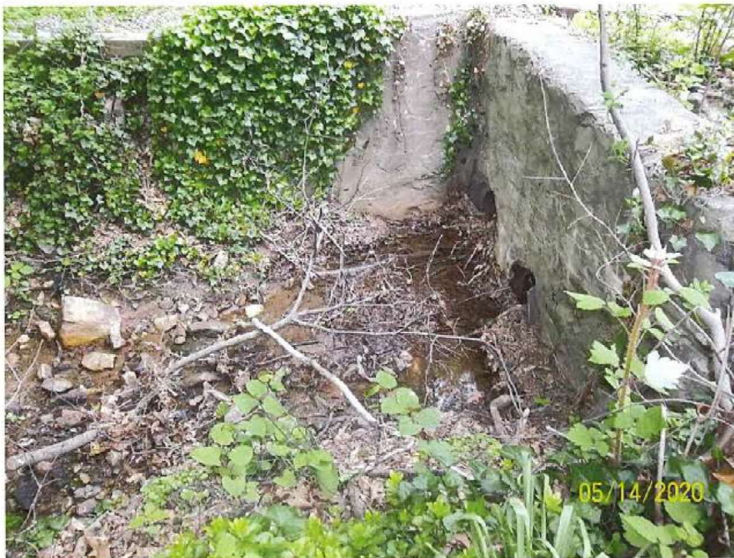
Figure 17. A small branch splits from Pine Ridge Run near the intersection of Beechwood Road and Pine Ridge Road. Flowing water is observed.
