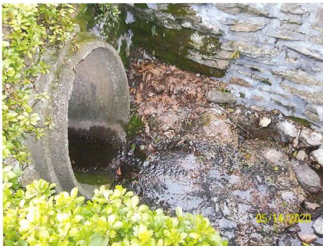
Figure 10. Culvert on the other side of Meredith Drive where Pine Ridge Run resurfaces.
