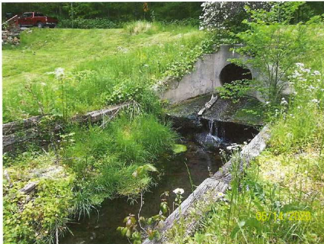
Figure 12. Culvert on the other side of Turner Road where the Tributary resurfaces.
