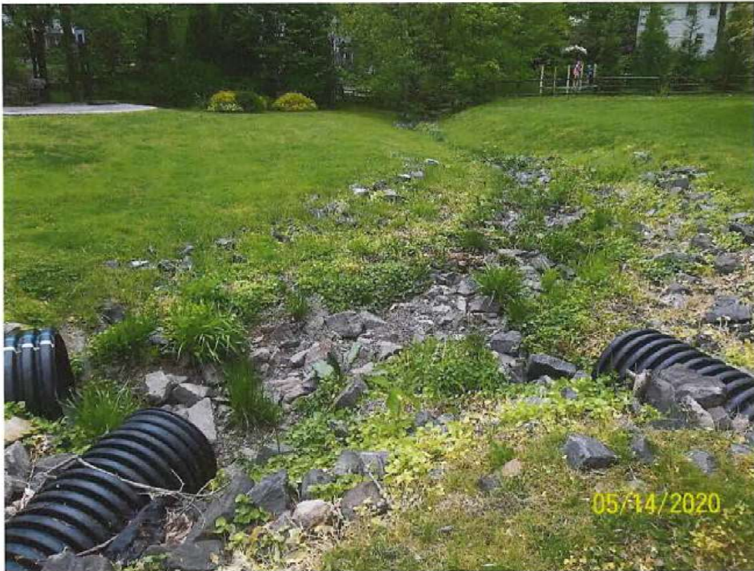
Figure 3. Closer image of pipes from Figure 2. No flowing water present.
