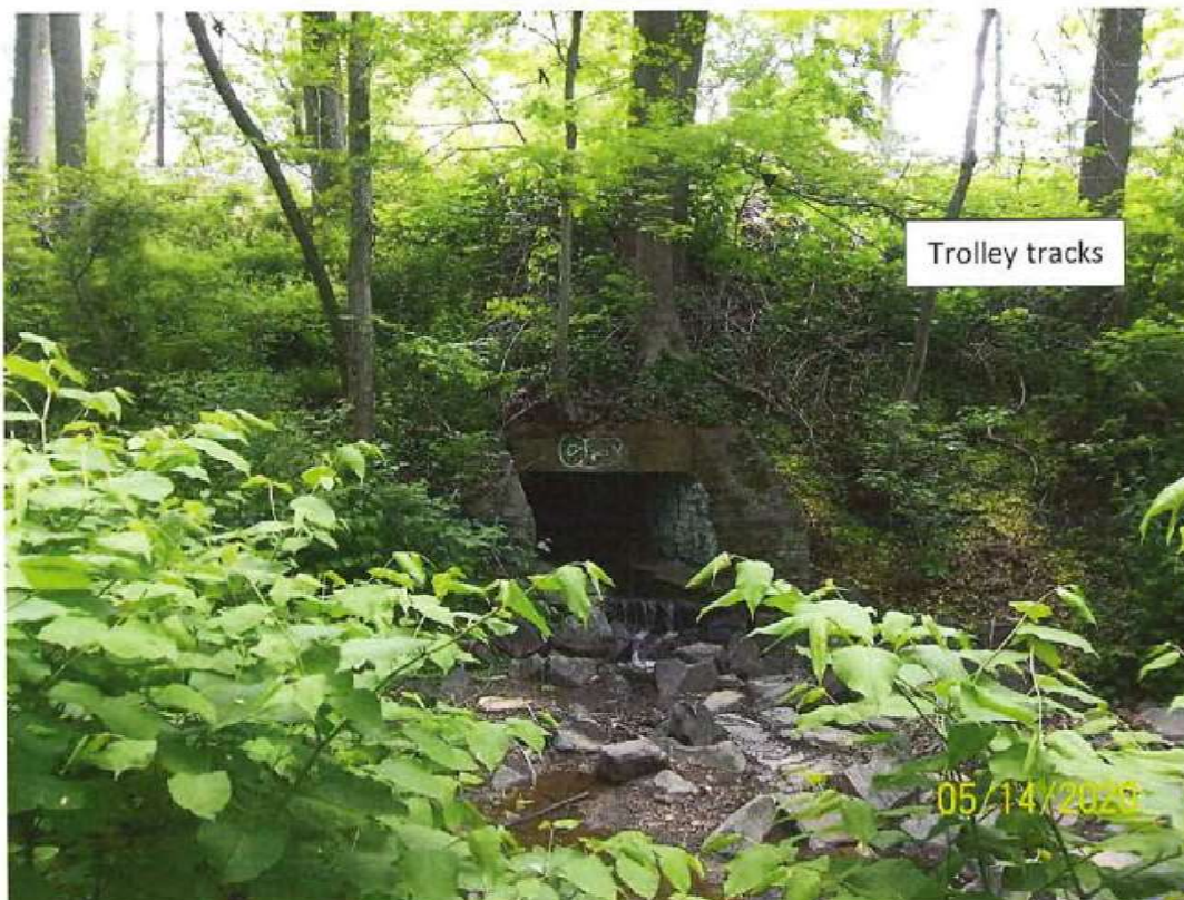
Figure 30. Pine Ridge Run resurfacing from culvert on the other side of the trolley tracks.
